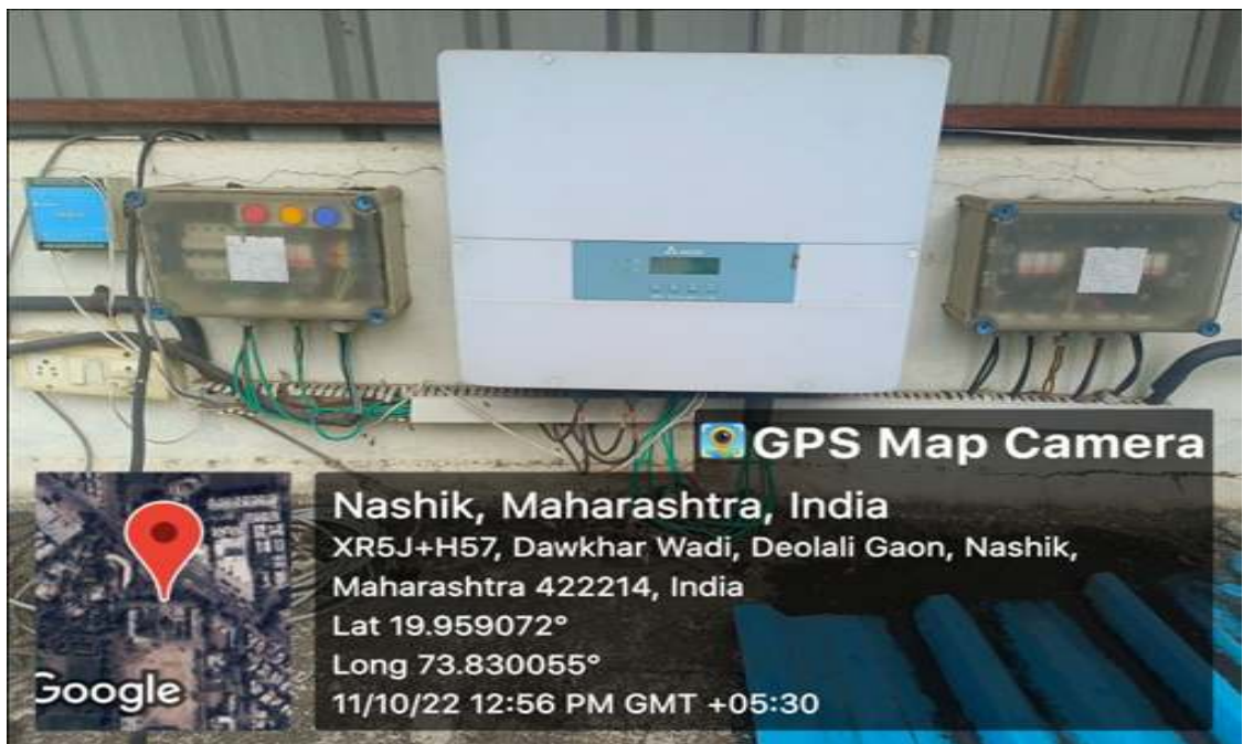
Solar Energy converter
