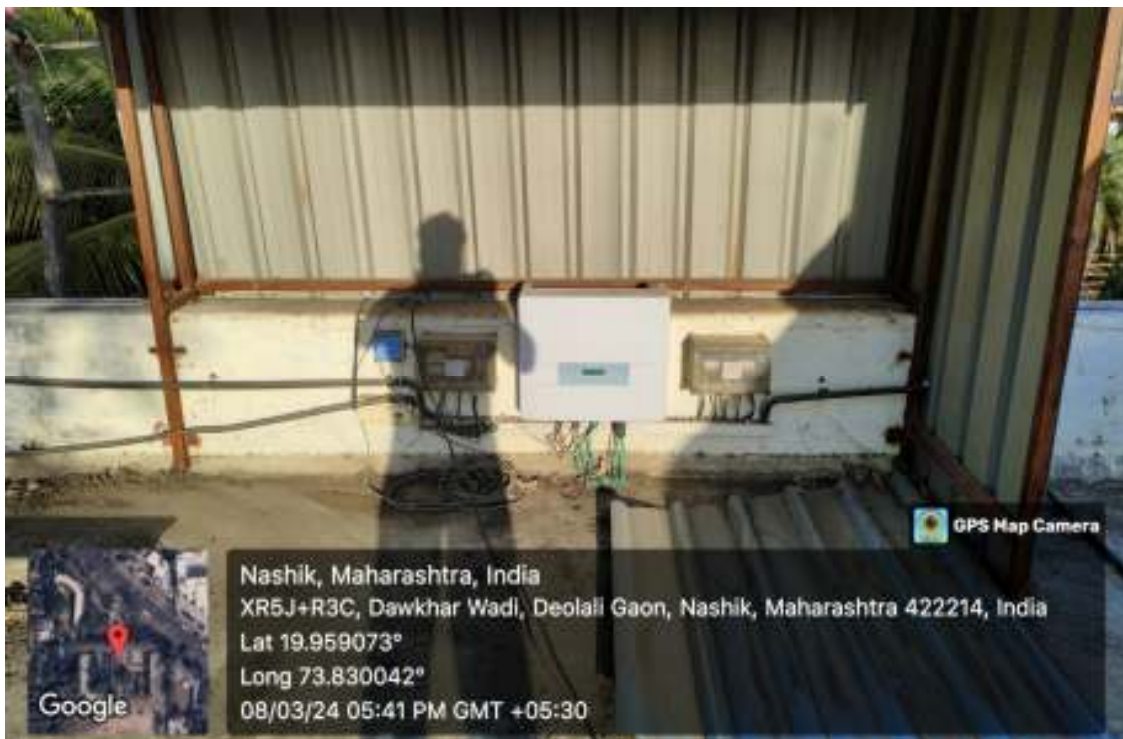
Solar Energy converter
