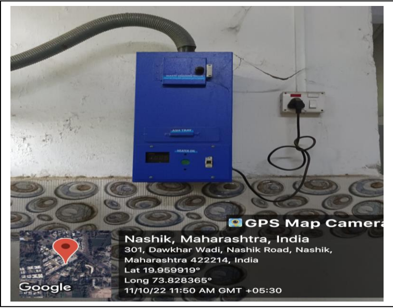
Girls Common Room—Sanitary Pad Disposal machine
