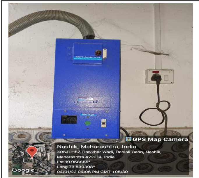
Girls Common Room—Sanitary Pad Disposal machine
