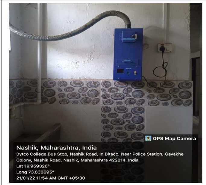
Girls Common Room—Sanitary Pad Disposal machine
