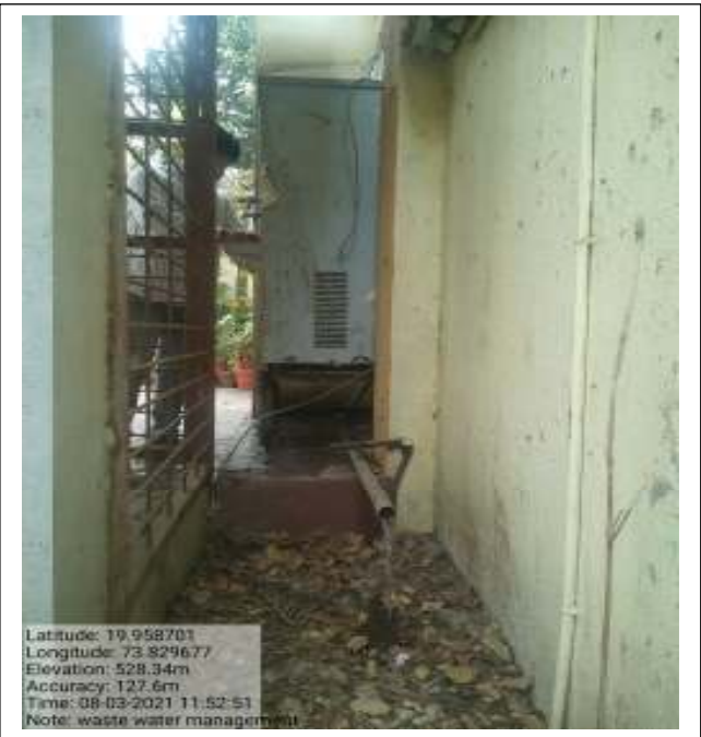
Waste water recycling
